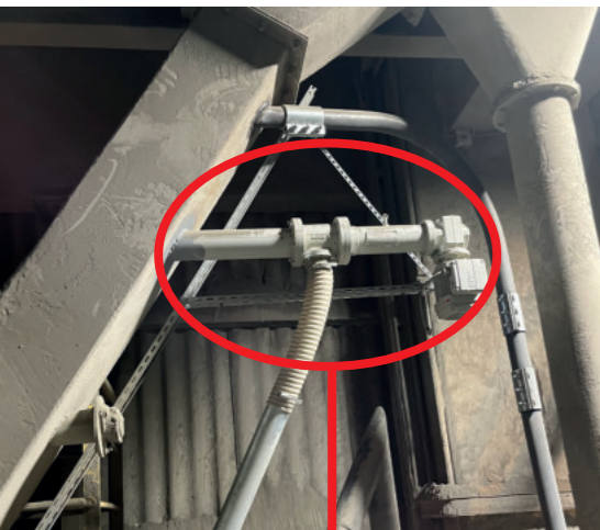
Installed Screw Sampler
